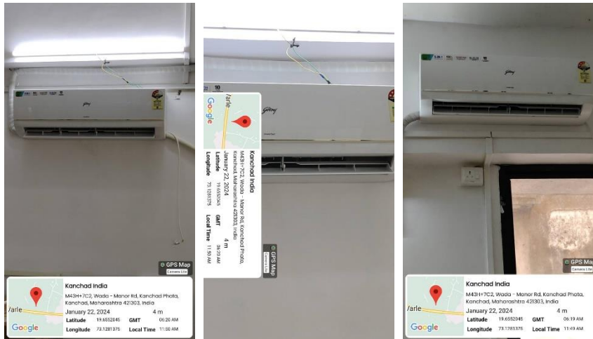
AC in the rooms
