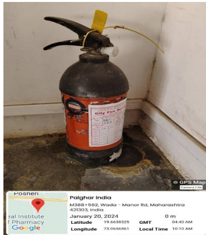
Fire Fighting System is installed
